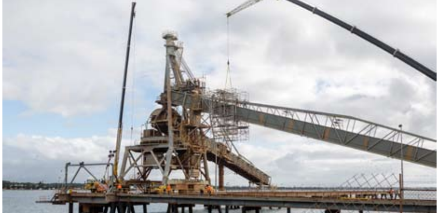
A 220 tonne was required to complete work at the top of the berth three ship loader.
