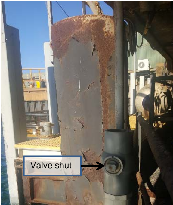
Figure 2 Berth outlet valve shown in closed position to divert water to tanks
