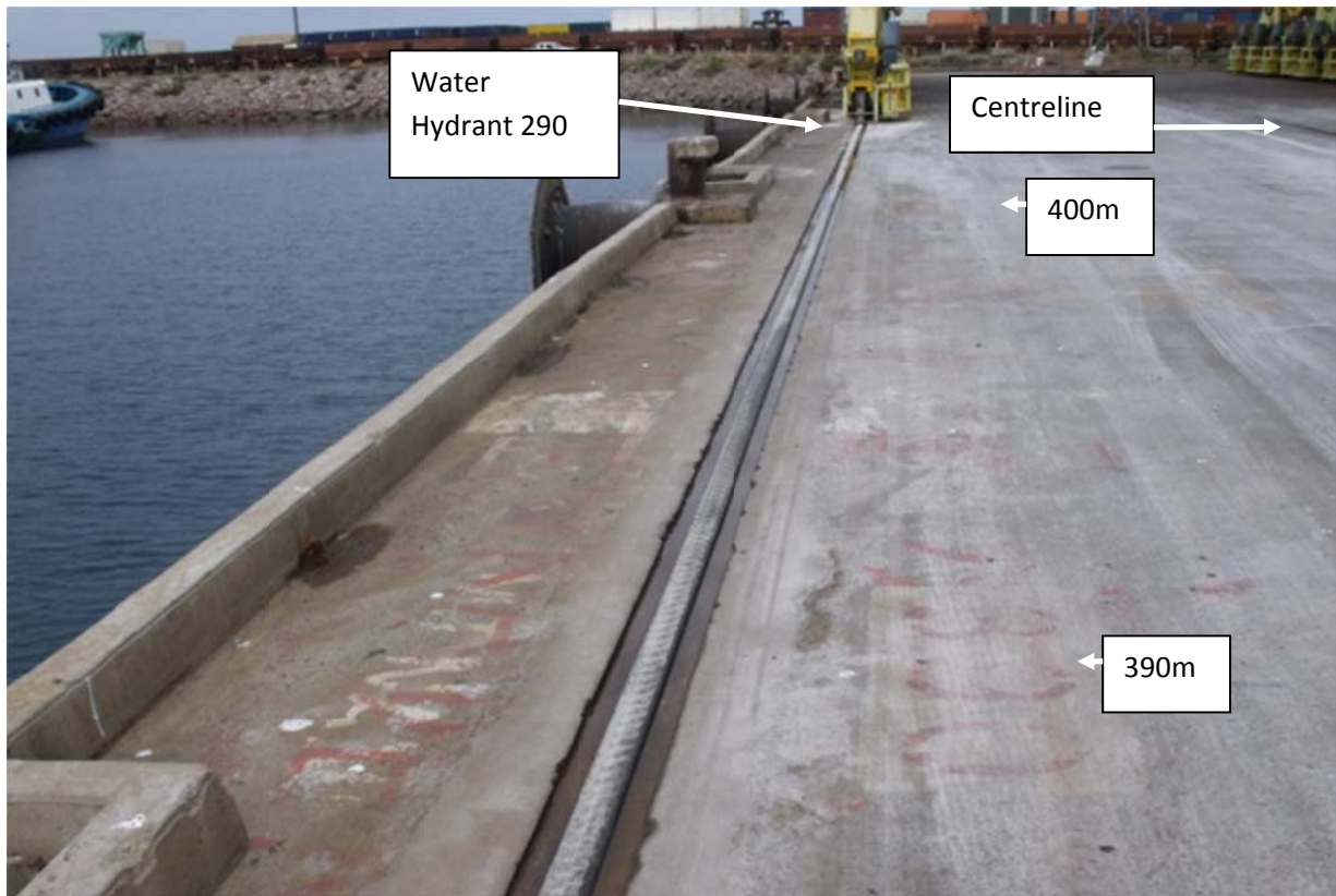
Figure 7. Alignment of hopper washdown between 390 to 400m mark on berth 2, landward of berth centreline. The area shown should be kept clear to allow Environmental Services to sweep up any washings that escape the containment used to capture hopper washings.
