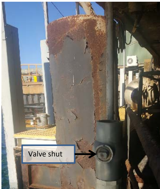
Figure 1 Berth outlet valve shown in closed position to divert water to tanks
