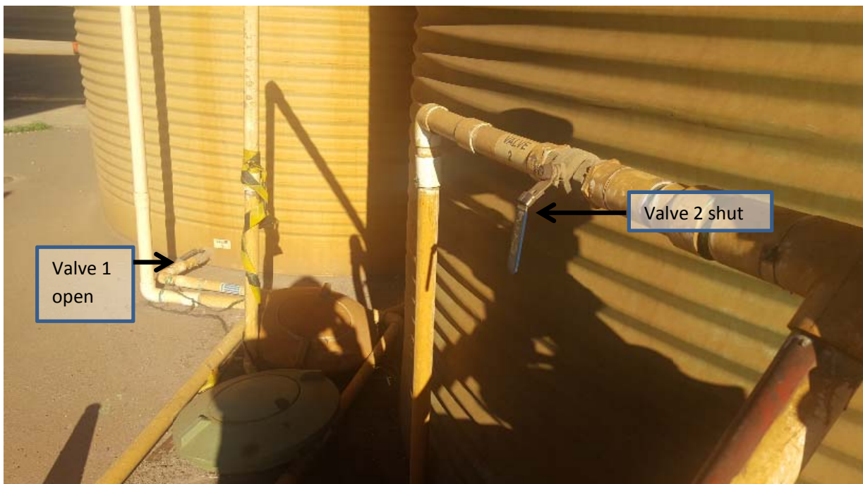
Figure 2 Valves 1 and 2 in position to divert Berth 2 run-off to the empty wastewater tank
